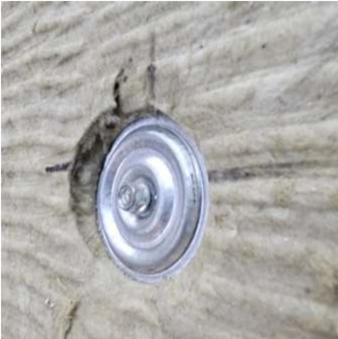
Plate 1 – Metal Washer Embedded Deeper Following Testing (1)
