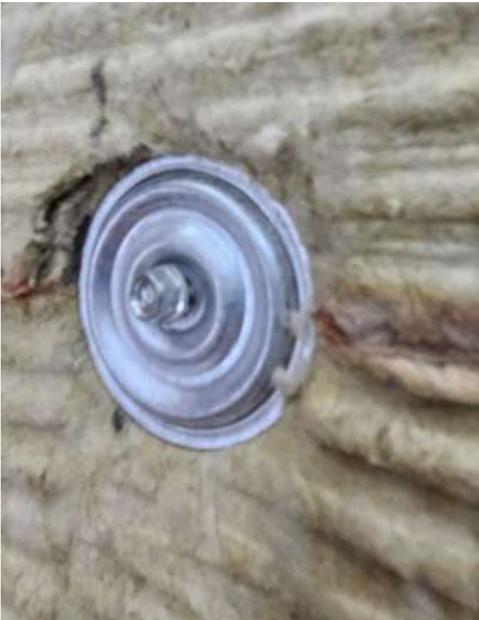
Plate 2 – Metal Washer Embedded Deeper Following Testing (2)
