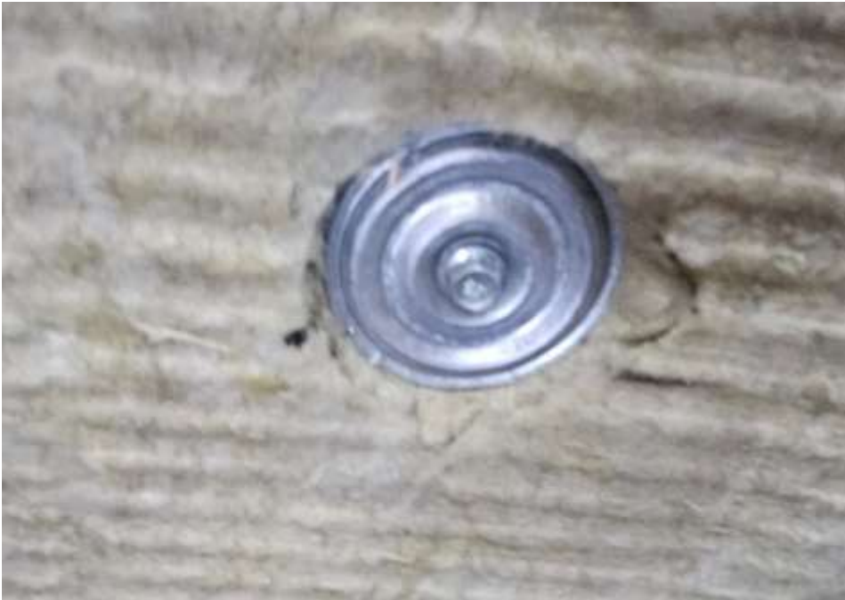
Plate 3 – Metal Washer Embedded Deeper Following Testing (3)
